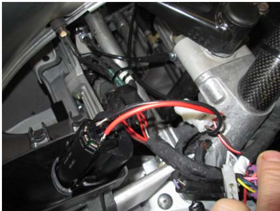
29. Use a 12 volt battery and power the pump to ensure water is pumping. You should be able to hear the pump running, let the pump run for 30 to 45 seconds.
